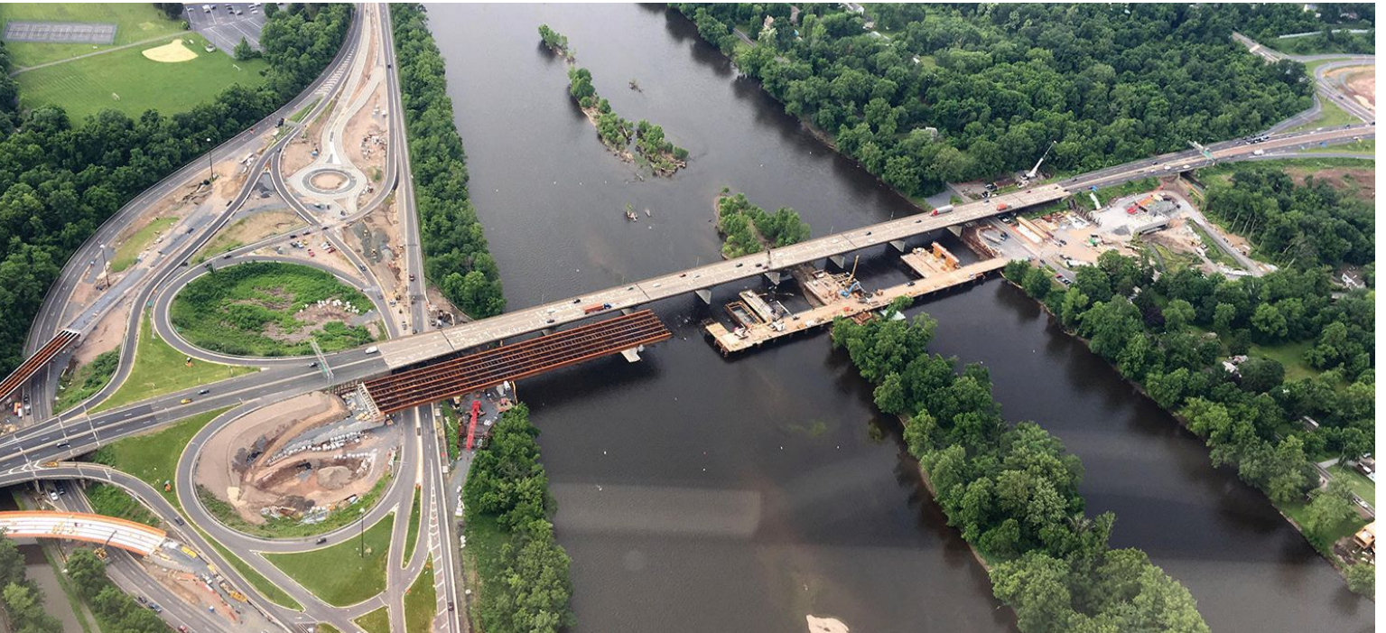
Scudder Falls Route 29 Interchange looking towards Pennsylvania. Photo credit: Michael Baker International
