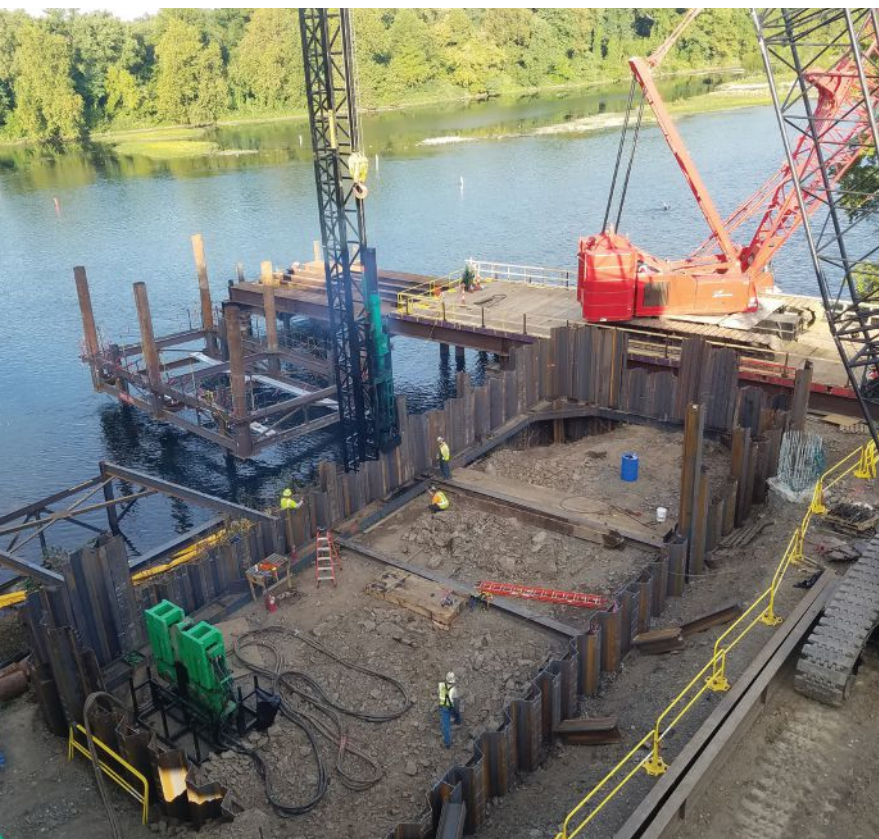
A decade-long environmental documentation process preceded design and construction. Photo credit: Michael Baker International
